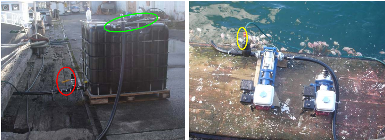
Figure 2.8: IBC header tank, hoses and hose fittings established on the wharf (left). Pumps secured near sea-level on finger punt positioned below the wharf (right). Lowara SV205 T304 (left) and CO350/03 (right).
