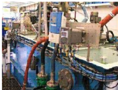
Figure 11 AHCS Effluent Water Treatment System
